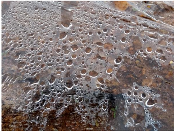
Plate 3. Moisture trapped inside the transparent poly-coated layer.
